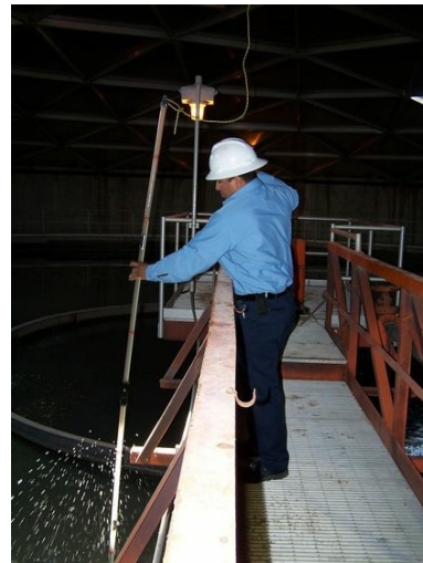
EPWater is accelerating maintenance at the Haskell Street Plant to reduce odors.
